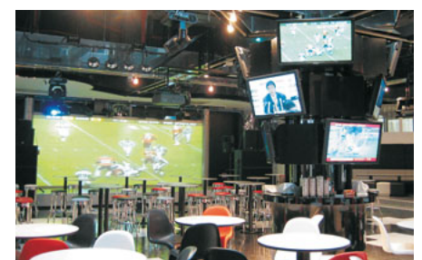
Plasma displays installed on the pillar (right) and two 150-inch screens (left).
