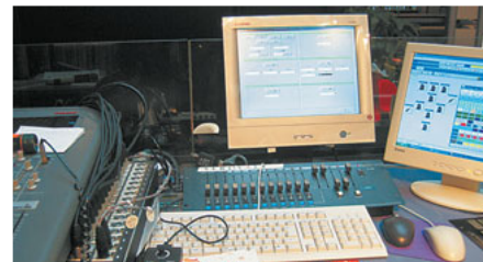
Control PC installed in the DJ booth simplifies control of a wide range of input and output sources.
